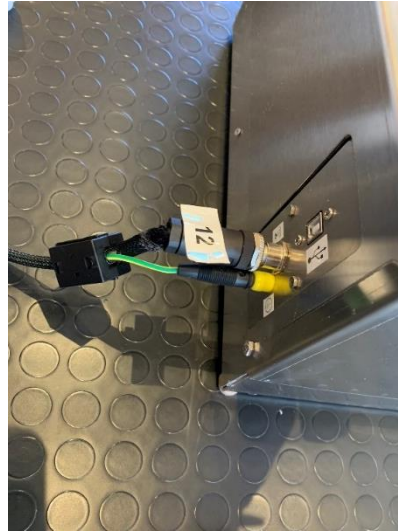
Figure 4.20. Connection of the earth wire of the ABU sensor pack cable to the ABU ventilator.
