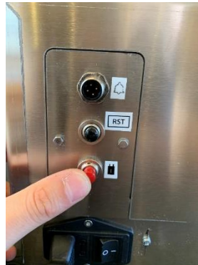
Figure 6.2. Turning on ABU ventilator using the internal battery
